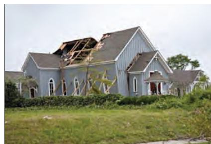
Wooden Church after Tornado Damage (Source: stock photo)
